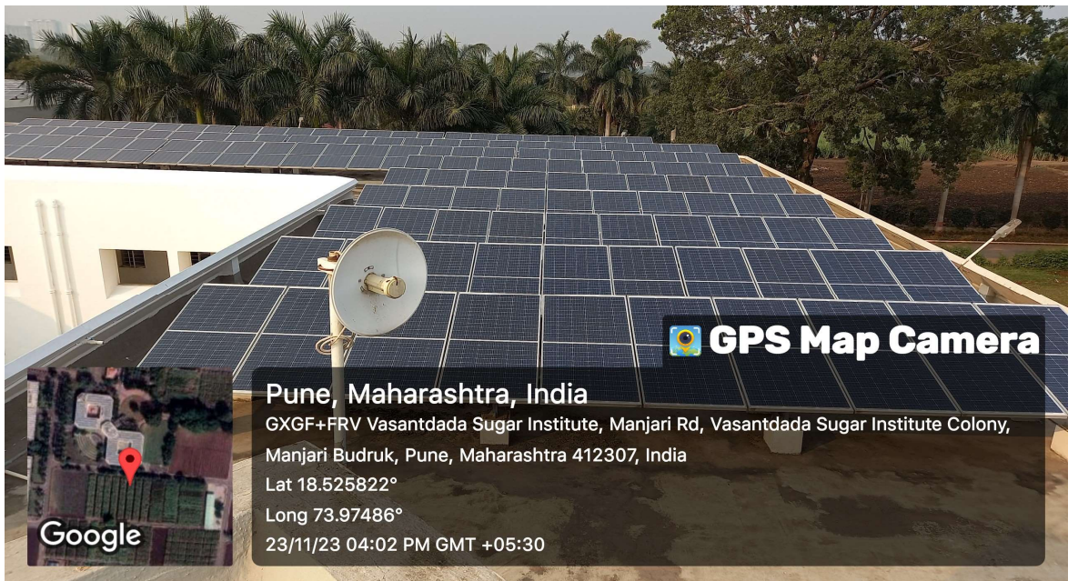
Service Provider Antenna
